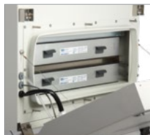
Redundant Exhaust HEPA Filters (Quantity 2)
